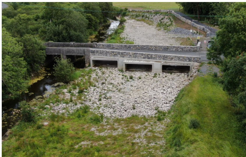
Figure 3: Completed Works at Rinn Bridge (3 new flood eyes on right hand side)
